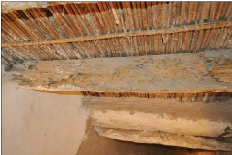
Figure 3: Biological decay of palm in the OCG Source: Municipality of Ghadames City, Libya
